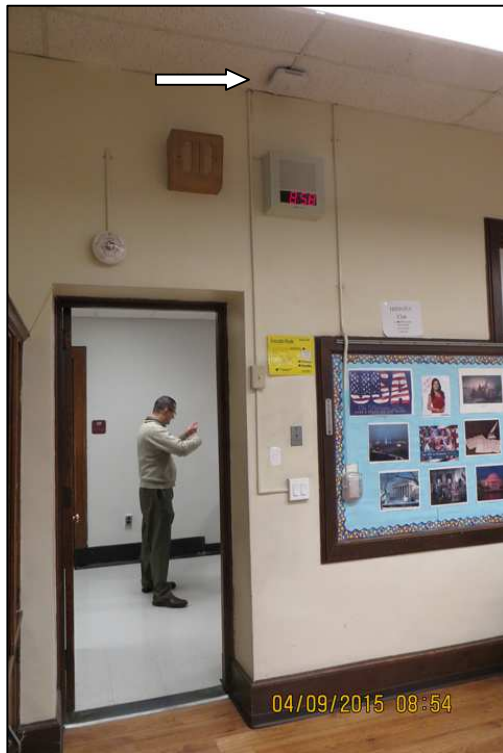
Room 204 – Classroom (antenna on ceiling)
