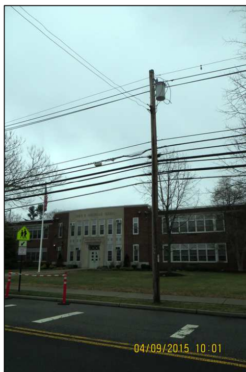
Power line transformer on utility pole in front of school
