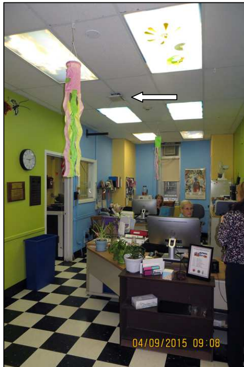
Principal's Office – antenna on ceiling (arrow)
