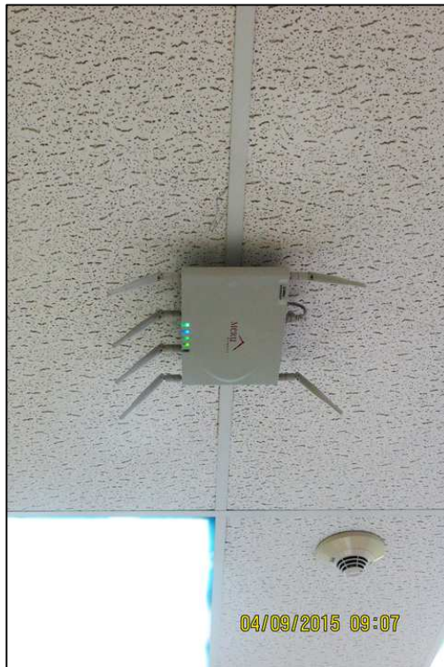
Principal's Office – close-up of antenna
