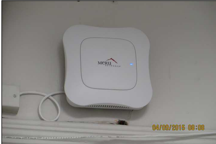
Principal's Office – close-up of antenna
