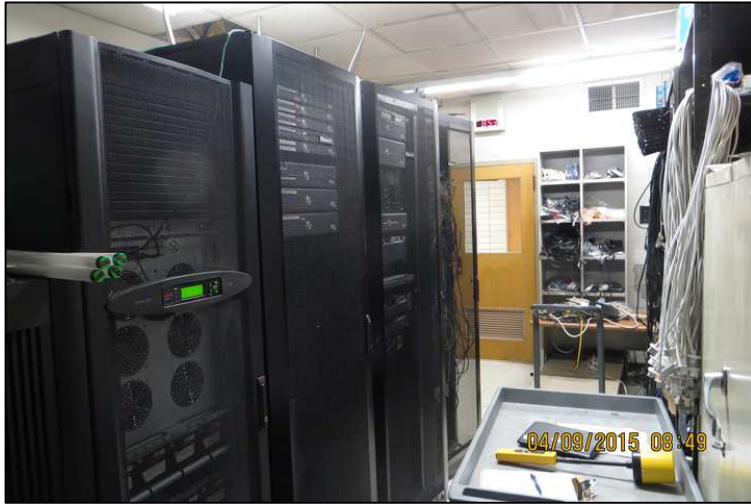
MDF – Server Room (no antennas)
